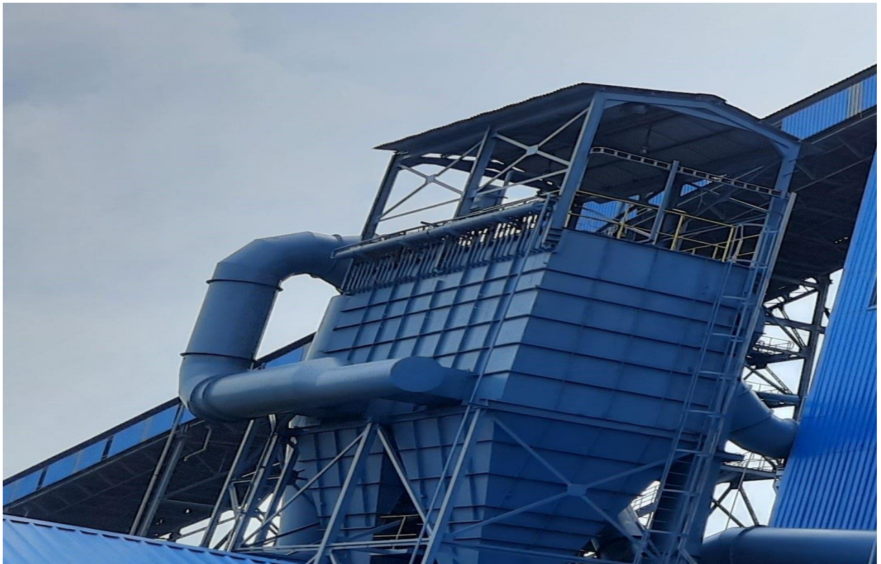
DUST EXTRACTION SYSTEM AT TRANSFER POINTS
